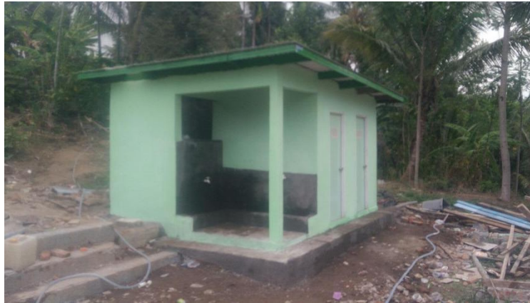
Permanent sanitary facility
